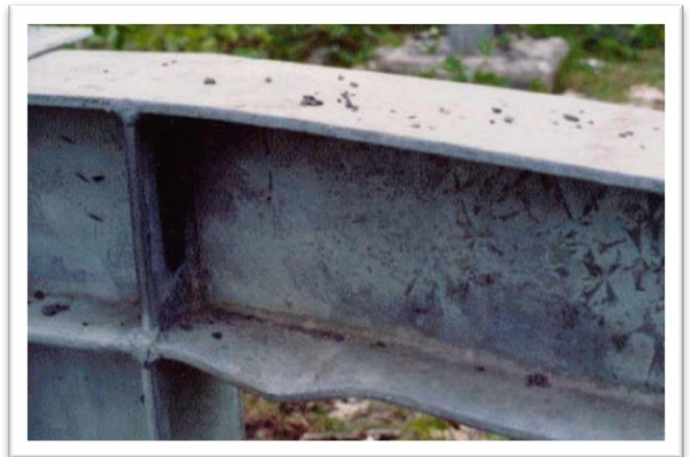
Flange Local Buckling Example
