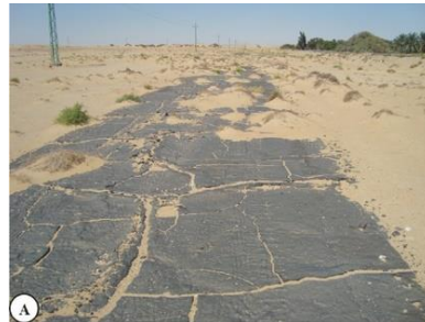
Destructive effect of sand dunes on asphaltic road
