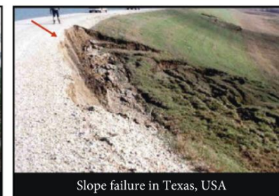
Slope failure in Texas, USA
