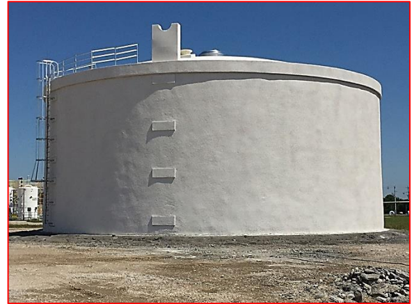
CIRCULAR RESTING ON GROUND TANK
