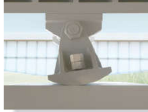
The rocker support for this bridge girder allows horizontal movement so the bridge is free to expand and contract due to a change in temperature. (4)
